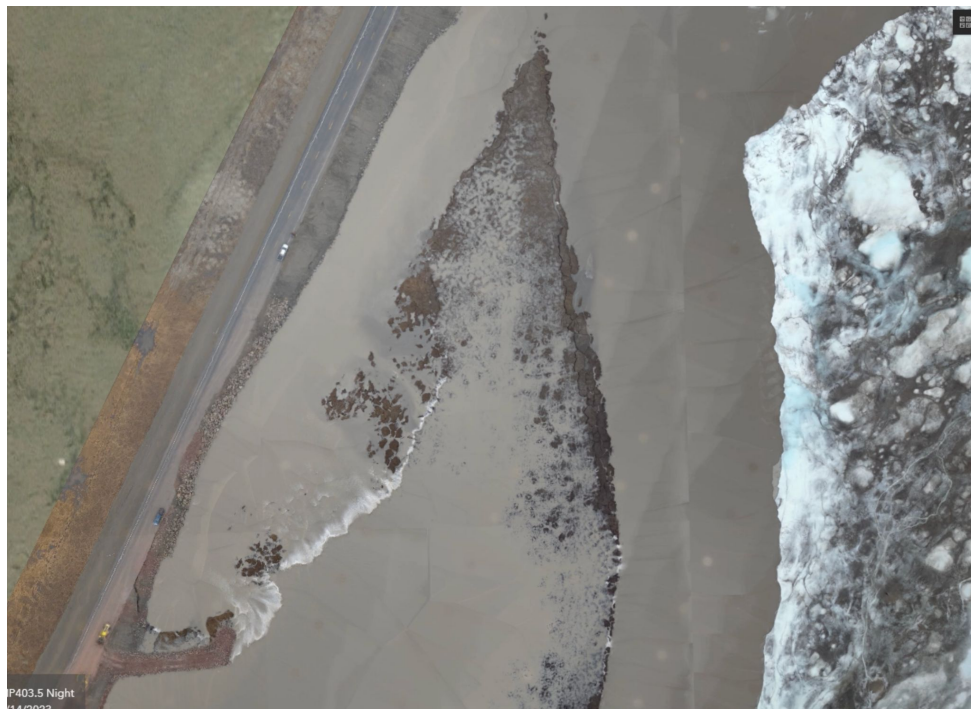
Dalton Highway erosion June 14th AK DOT Drone
