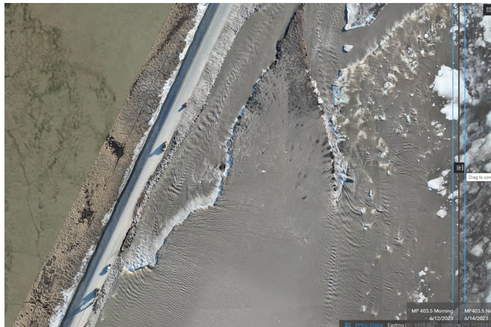
Dalton Highway erosion June 12th AK DOT Drone
